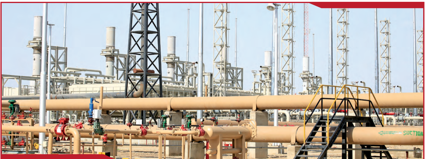
Major achievement: A view of HQ-2 Daur where the Company has installed 6 turbo compressors
