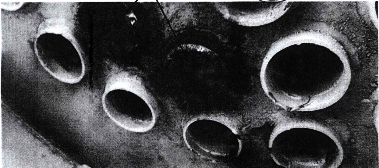
Leaked Heat exchanger pipes blocked bottom side
