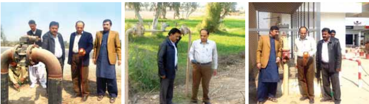
A new CP Station at Shandan Mori near Qazi Ahmed on main National Highway Road was commissioned in February 2014 by Nadeem Ahmed Memon, Sr. Engineer (CP) under the supervision of Naik Muhammad Shaikh, DCE In-charge (CP) for cathodic protection of Bari supply main and enroute villages.
